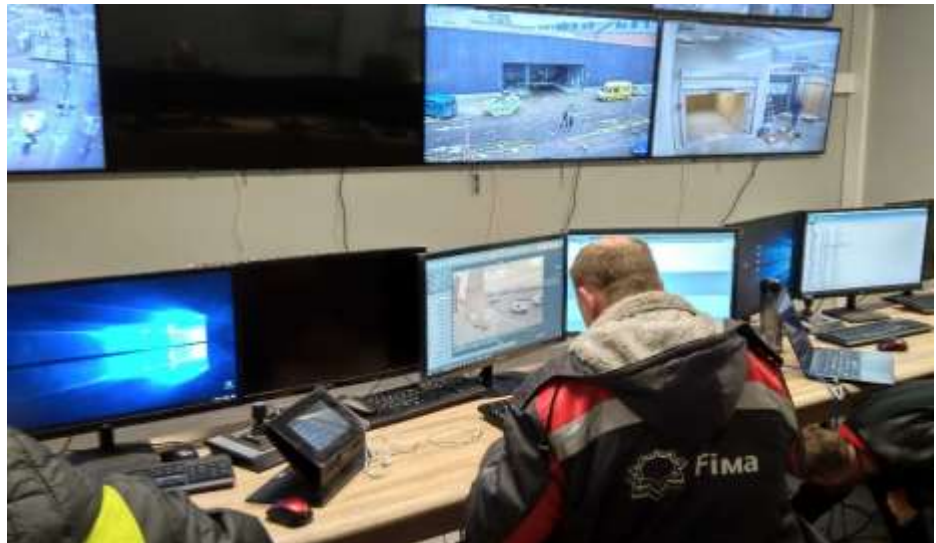
Illustration: SIA Fima engineers preparing security system for operation at Akropole. Source: Midpoint Security
